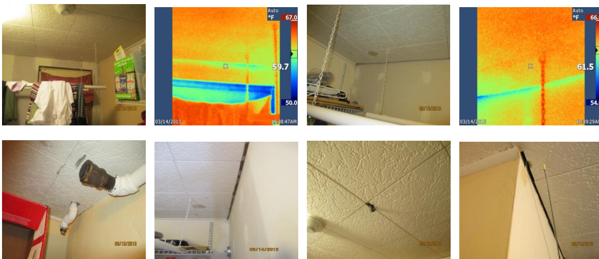
Examples of infiltration and loss at unsealed joints and penetrations in the Laundry area.
