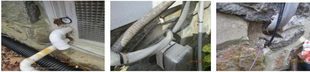
Examples of deteriorated seals at penetrations.
