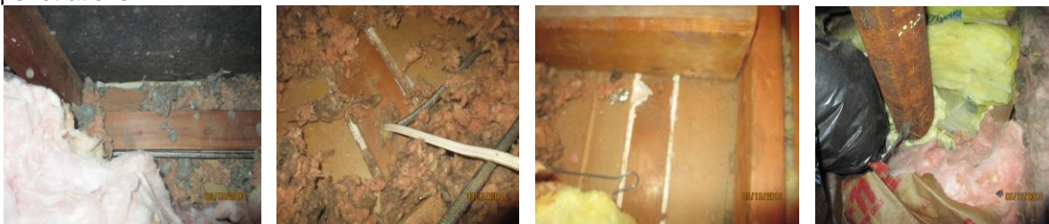
Examples of sealed top plates and penetrations.
