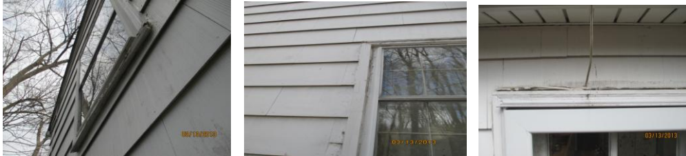
Examples of deteriorated caulk at windows.
