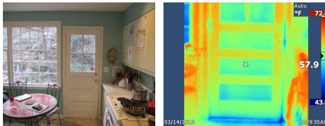
Kitchen door and TI indicating infiltration & loss.
