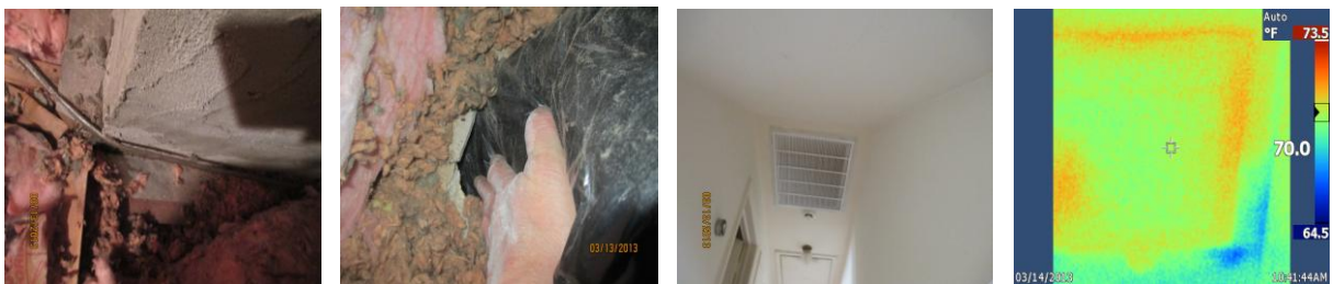
Examples of unsealed chimney and duct penetrations and TI showing example of loss at a RA vent.
