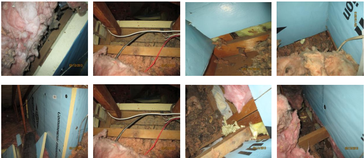
Unsealed top plates, joints, and breaks in the vertical wall at Kitchen soffit connecting the 2 attics.
