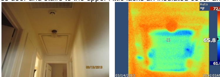
Loss at access stairs.
