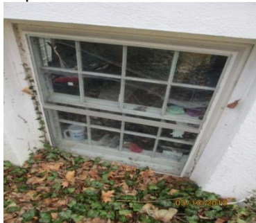
Storm window with cobwebs. Also sets at grade.
