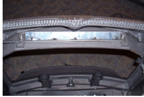
FIG. 5 Remove Primary Air Shutter
