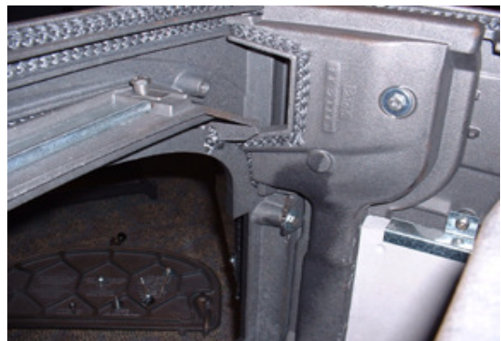
FIG. 4 Main Manifold Removed
