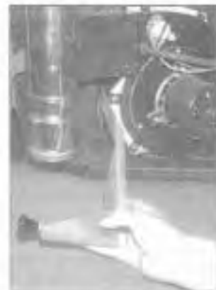
PHOTO A (damper position behind firebox)
